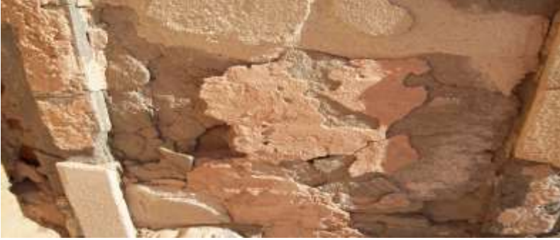
Fig. (17 ) deteriorated of plasters
