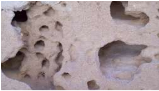
Fig. (9 ) Erosion of limestone by weathering are the principle factor of honeycomb and damage of limestone
