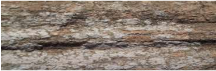
Fig. (16) biodeterioration of plasters.
