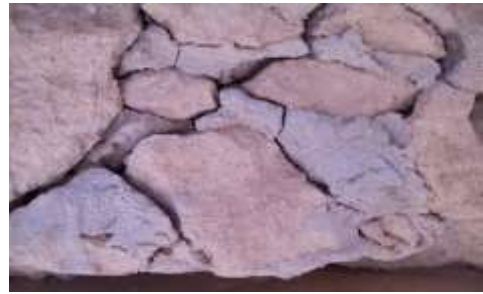
Fig. (10 ) Deterioration and disintegration of unsuitable mortars .
