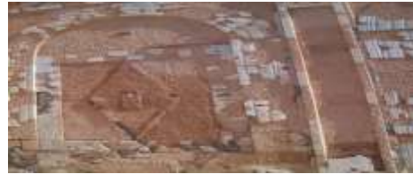
Fig. (12 ) Spallation of marble decoration slabs
